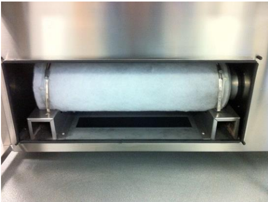
Installed Active-Carbon Filter
